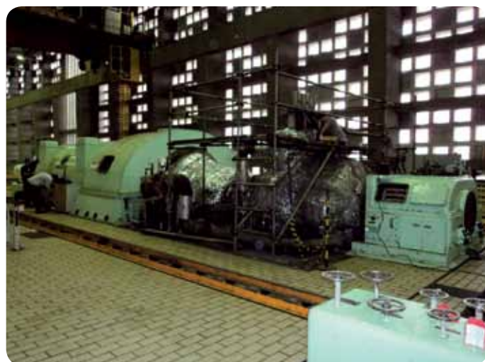
Adjusting the downholder bolts of the medium pressure turbine stator minimized vibrations, making it possible for the Brazilian power plant to resume operation at practically nominal steam temperature.
