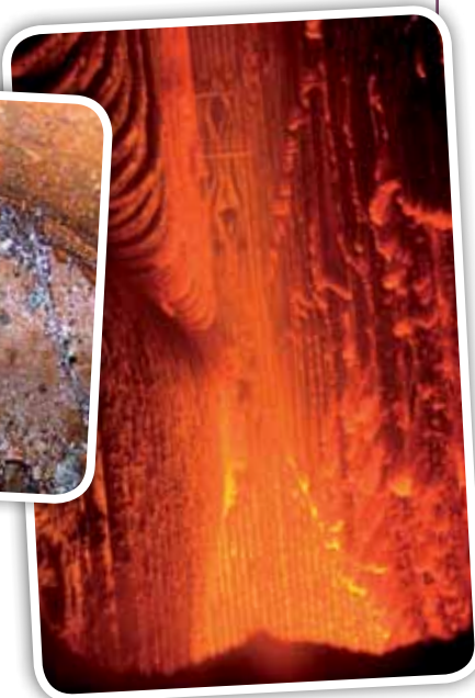
Severe slagging inside a boiler
