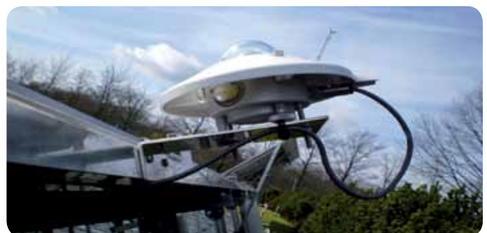
Laborelec is able to measure the intensity of sunlight using a pyranometer. This is an important parameter in accurately calculating PV performance.
