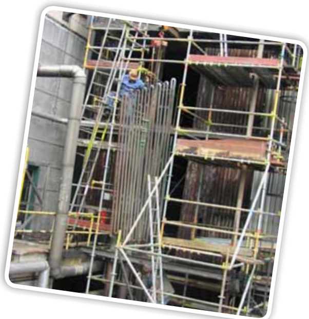
Laborelec assists in the selection of the most appropriate non-destructive testing technique to ensure a quick and efficient intervention on your boiler.
