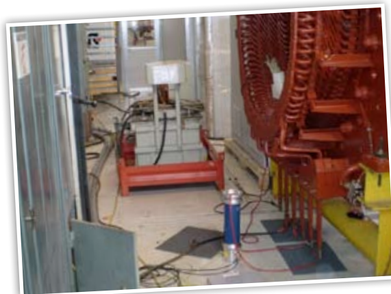
Our experts carried out partial discharge tests to identify the precise type of insulation wear.
