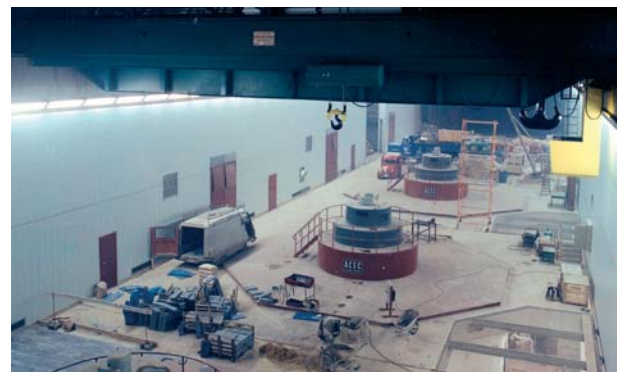
Engine room of a hydraulic power plant
