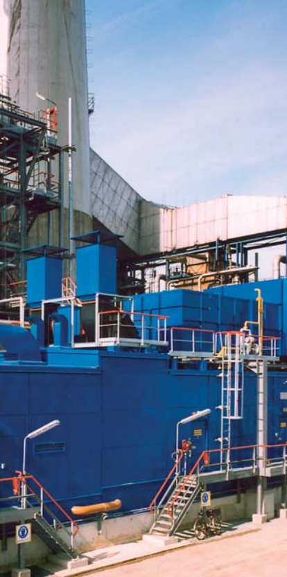
The 40 MW combined heat and power unit at the Esso site in Antwerp (Electrabel, Belgium).
