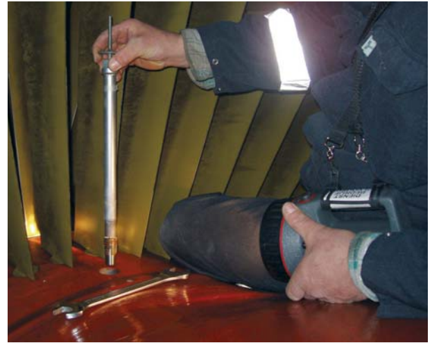
Placing a 170 gr weight at the compressor inlet during a balancing campaign of a gas turbine.
