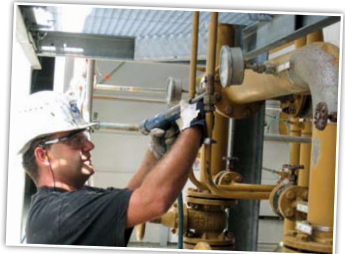
Removing rust during surface preparation is critical in ensuring a long paint lifetime.
