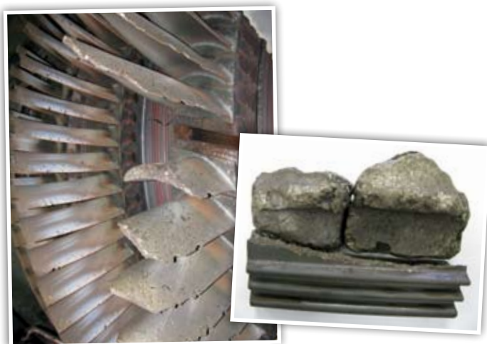
A broken rotor blade caused significant damage inside the gas turbine at the Rosen power plant. The insurance company reimbursed the repair costs based on the investigative results of Milan University and Laborelec.
