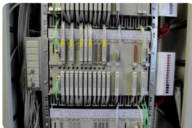
The LSTS is directly connected to the turbine controller.
