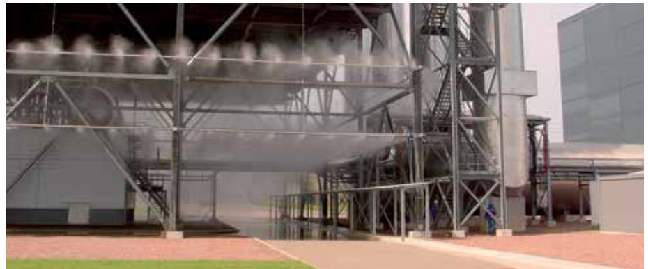
After implementing improvement actions, such as the spraying system of the air-cooled condenser at the Saint-Ghislain and Esch-sur-Alzette combined cycle gas turbine power plants, ENGIE Laborelec also performs comparative analyses. The return of experience is shared across the Group.
