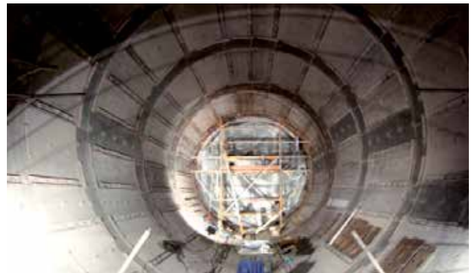
Flue gas duct
