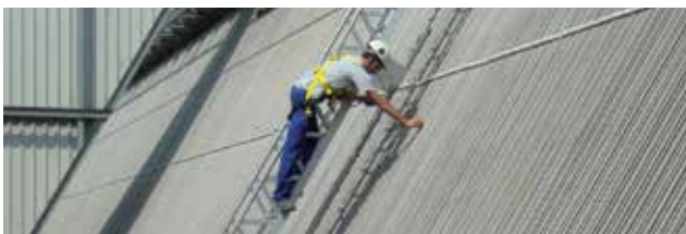
Wall and coating thickness measurements on aero-condensers
